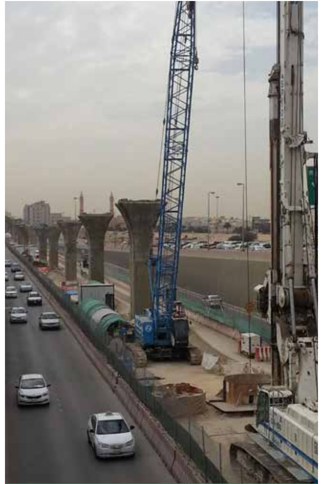
RIYADH METRO LINE2 MONOSHAF
